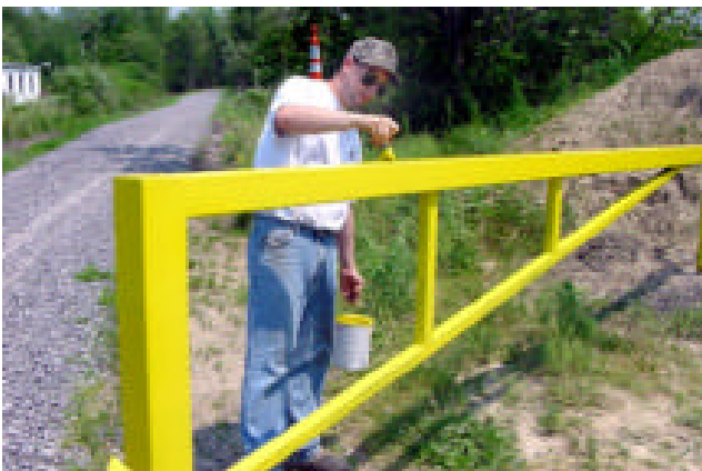
Dave Crino of Silver Creek, and Joe Rebman, seniors at the LoGuidace BOCES, installed two trail gates in Brocton. Here Dave Crino paints a gate they installed.
